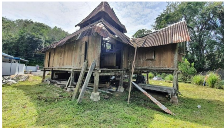
Figure 3: The oldest heritage masjid in Negeri Sembilan (Masjid Parit Istana) built in 1796. (Source: Author, 2021)
