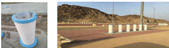
Figure 4.7: Water fountain stop point provided for the use of pilgrims
