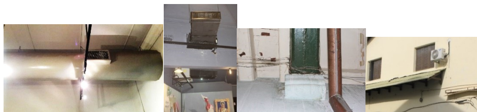
Figure 5: Intrusive installations, exposed electrical wiring and improper placement of air-conditioner compressors on building façade were among the inappropriate physical interventions found on building services element.
