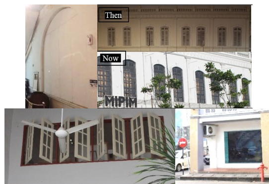
Figure 4: Fully enclosed original windows and replacement of non-harmonious modern windows were among the inappropriate physical interventions found on windows element.
