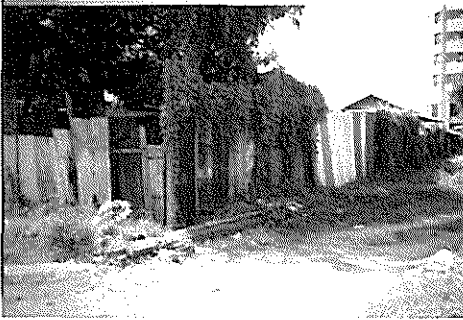
Photo C2.a: Zinc perimeter fencing – visual blight.
