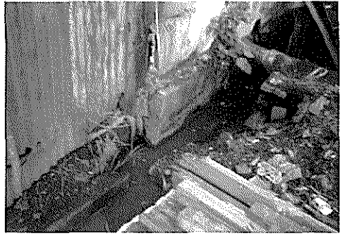
Photo C1.b: Clogged drain and zinc fence
