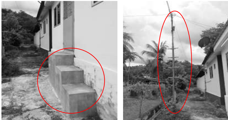
Figure 6: Stairs and utility poles become a tool for criminals to break into houses
