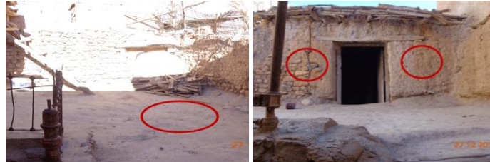
Figure 2 The floor condition at the yard (left) and exterior wall (right) Source: Author
