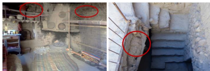
Figure 4 Poor condition of the common room walls (left) and stairs (right) Source: Author
