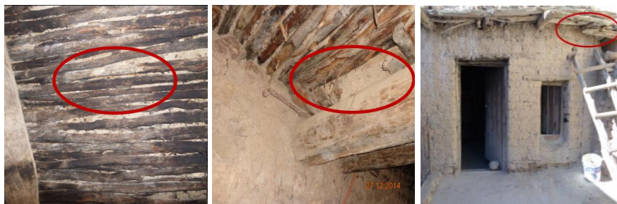
Figure 5 Deterioration of interior floors and partial structure collapse Source: Author
