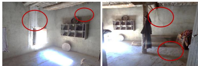
Figure 3 Cracks on the interior wall Source: Author
