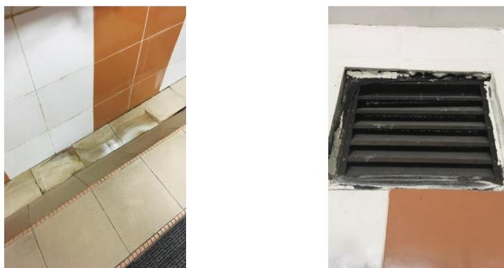
Figure 3 Unclean ducting system and stained floor, ablution room Gate-B Source: Author
