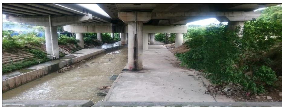
Figure 5: The neglected vacant space below AKLEH negligence devoid of specific function
