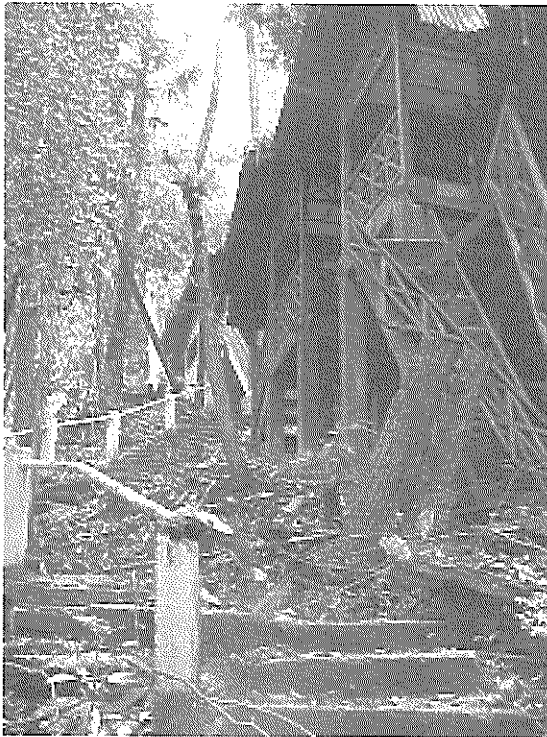
FIGURE 3: Chalets at this hill resort deteriorate without proper maintenance
